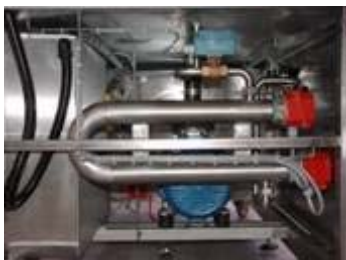
After rinse heater
