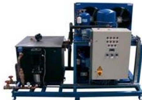
Low capacity water chiller, installed on one frame, inside the building.
