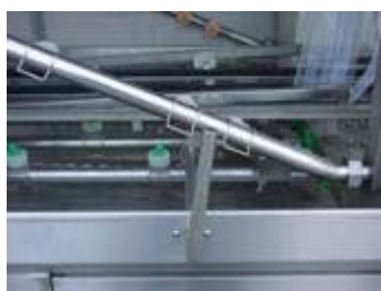
Mechanical transport stop
